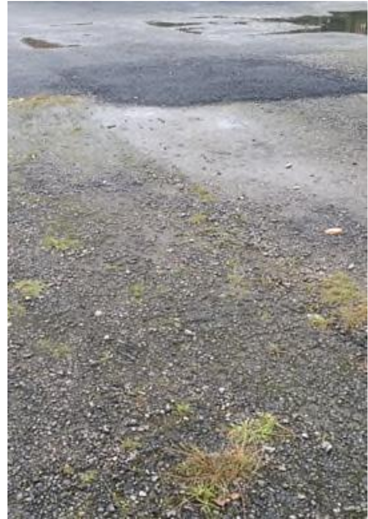
Uneven and mossy surface in the car park
